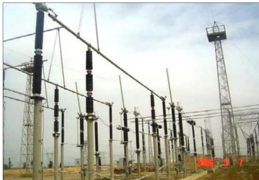
Rehabilitation and expansion of a 400kV/132kV substation along with the five feeders in the Diyala Province (2004).
